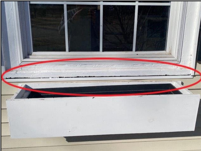
Paint and Caulking - deteriorated / missing
