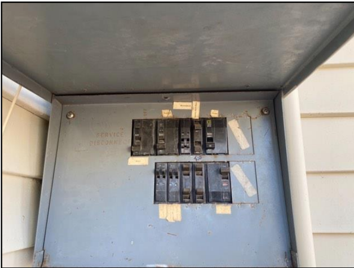
Breakers - exterior wall
