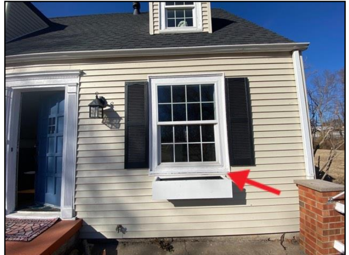
Paint and Caulking - deteriorated / missing
