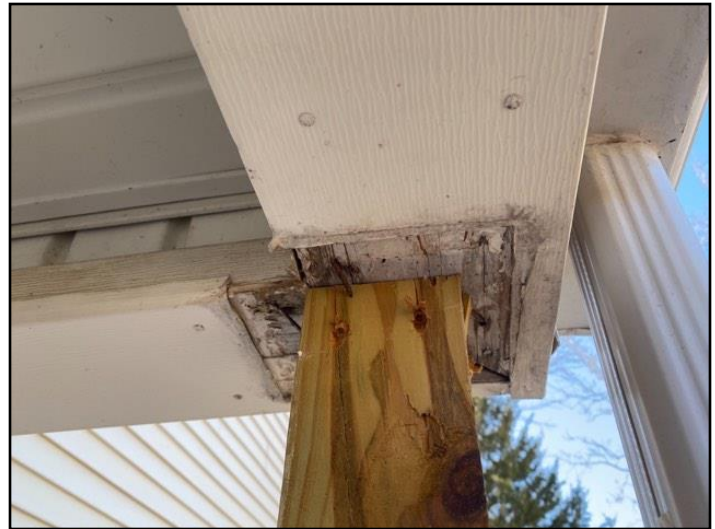
Poorly secured at top or bottom
